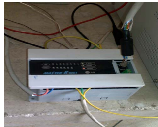
Fig. 18 PLC connected to tracking motor and drive card
