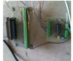
Fig.17 Data acquisition connected to computer
