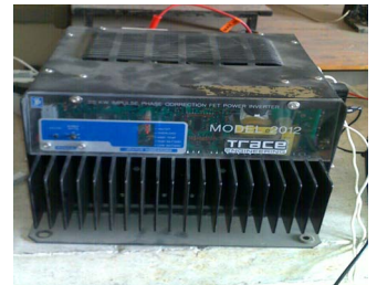
Fig.19 solar Inverter used.
